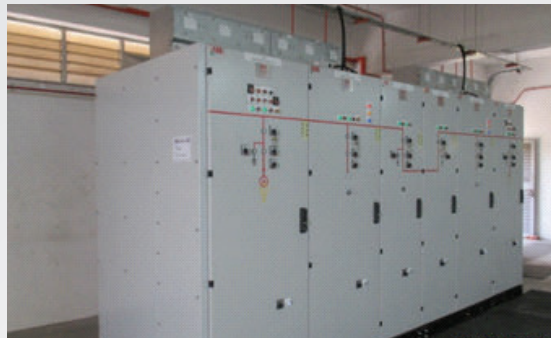
Selepas - Switchgear 33kV Gas Circuit Breaker (GCB)
