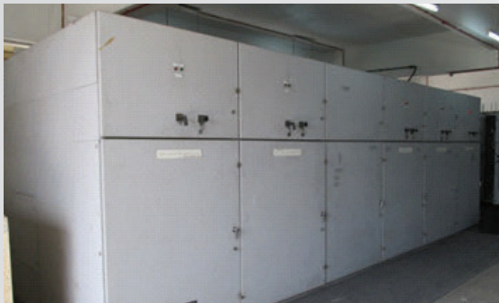
Sebelum - Switchgear 33kV Vacuum Circuit Breaker (VCB)
